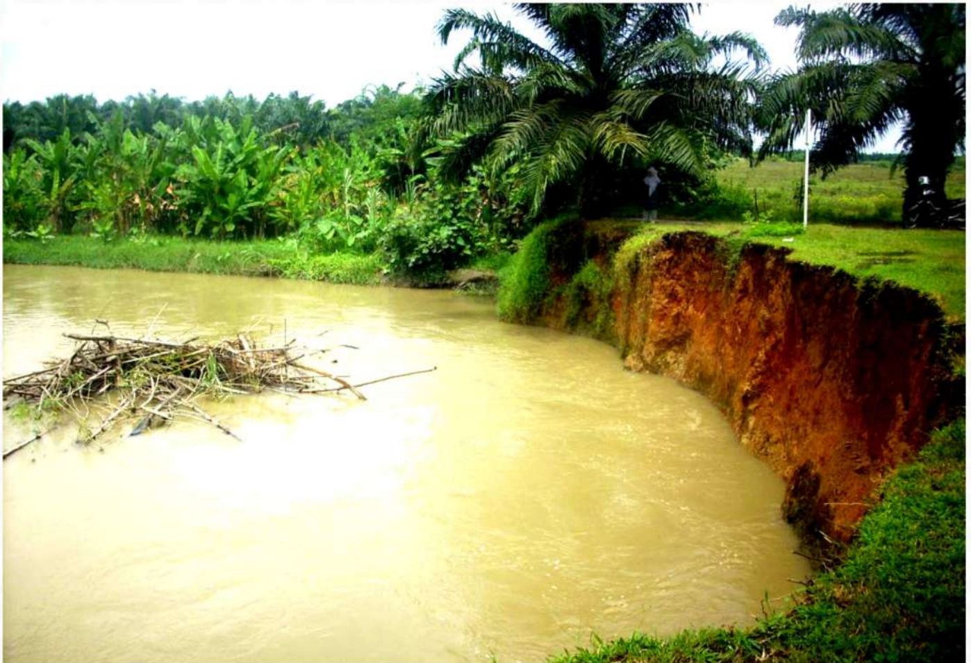
Gambar 14. Erosi tebing sungai ( streambank erosion )
