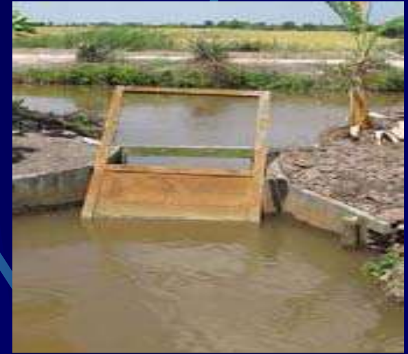
Pintu flapgate inlet
