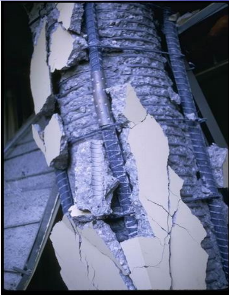
Detailed view of column with spiral confinement steel. The spiral confinement steel helped keep the concrete core intact. The longitudinal reinforcement is tied on the exterior of the spiral; this detail leaves the longitudinal steel vulnerable.
