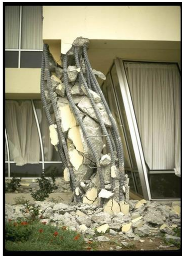
Example of damage to the corner columns at Olive View Hospital which was the result of poor seismic detailing. [9]
